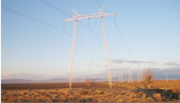
Guzar Surkhan Transmission Line, Uzbekistan, for export of electricity to Afghanistan
