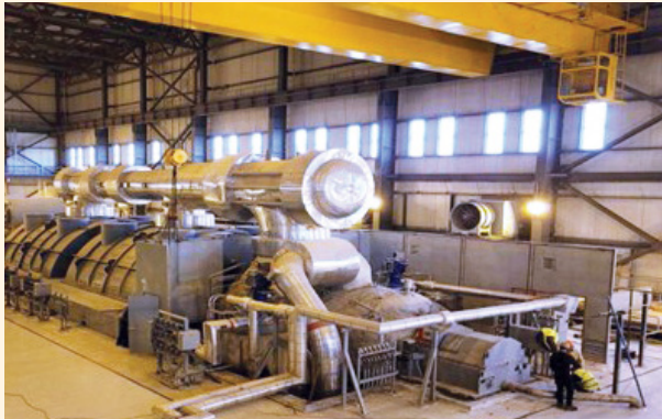
5: West Cairo Power Plant Project - Turbine and Generator 1
