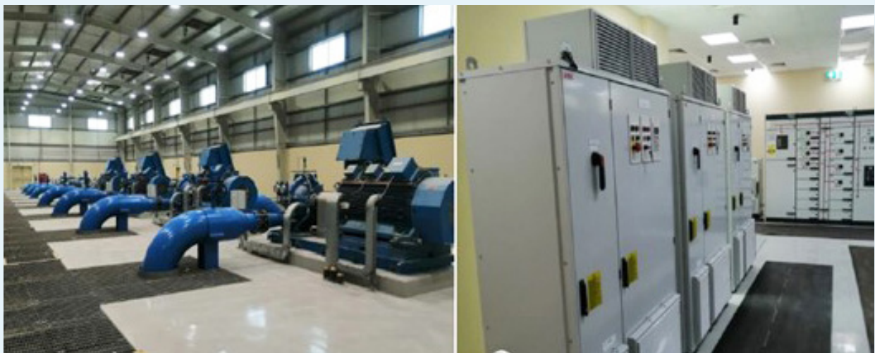
10: Pumps Hall in Sitra Forwarding Distillate Station FDS Variable Speed Pump/MEICA Room Sitra FDS
