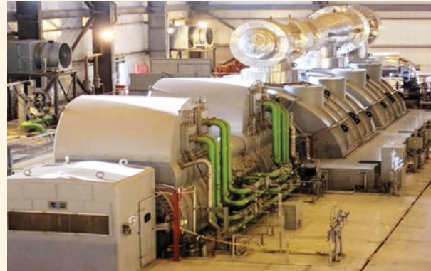
6: West Cairo Power Plant Project - Turbine and Generator 2
