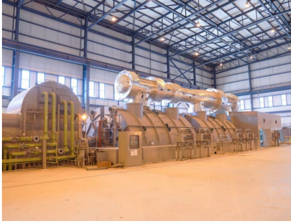
5: Steam Turbine Generator - Assiut (El-Walidia) Thermal Power Plant Project
